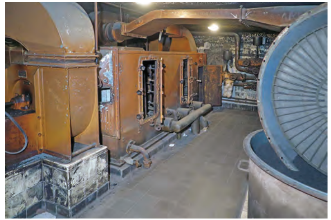
Ventilation Plant for the US Air Force bunkers beneath Tempelhof. Photo Clive Penfold
